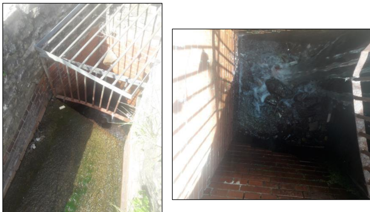
Figure 12: Image of 'Culvert Inlet 1' captured post event during CCTV surveying operations (30/07/2020) (left) and evidence of debris accumulation within the culvert chamber (right)
