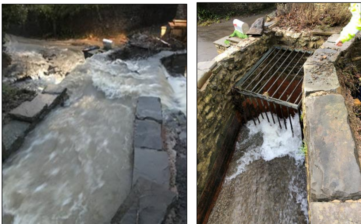
Figure 5: Evidence of 'Culvert Inlet 1' surcharging during the storm event and conveying southwards towards Column and Dumfries Streets (left) (image provided by resident), and 'Culvert Inlet 1' post storm event (right) (captured by RCT's Flood Risk Management team on 20 th February 2020)
