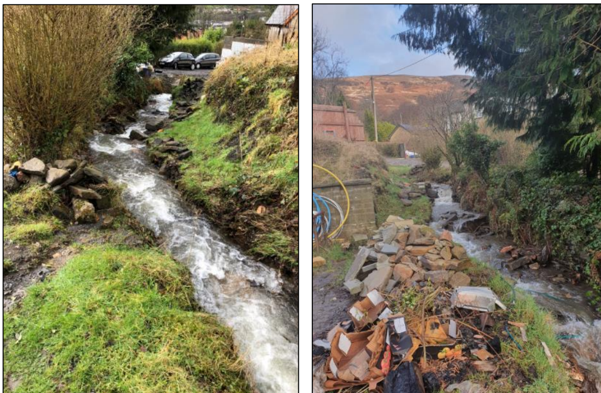
Figure 22: Unnamed open watercourse upstream of 'Culvert Inlet 1' showing evidence of large stones within the channel and surrounding embankment area (captured by RCT's Flood Risk Management team on 20 th February 2020). Looking downstream towards 'Culvert Inlet 1' (left) and looking upstream towards the outfall of 'Culvert Inlet 2' (right).
