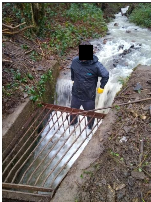
Figure 15: Photo of 'Culvert Inlet 3' following initial debris clearance by local residents on 16 th February 2020.
