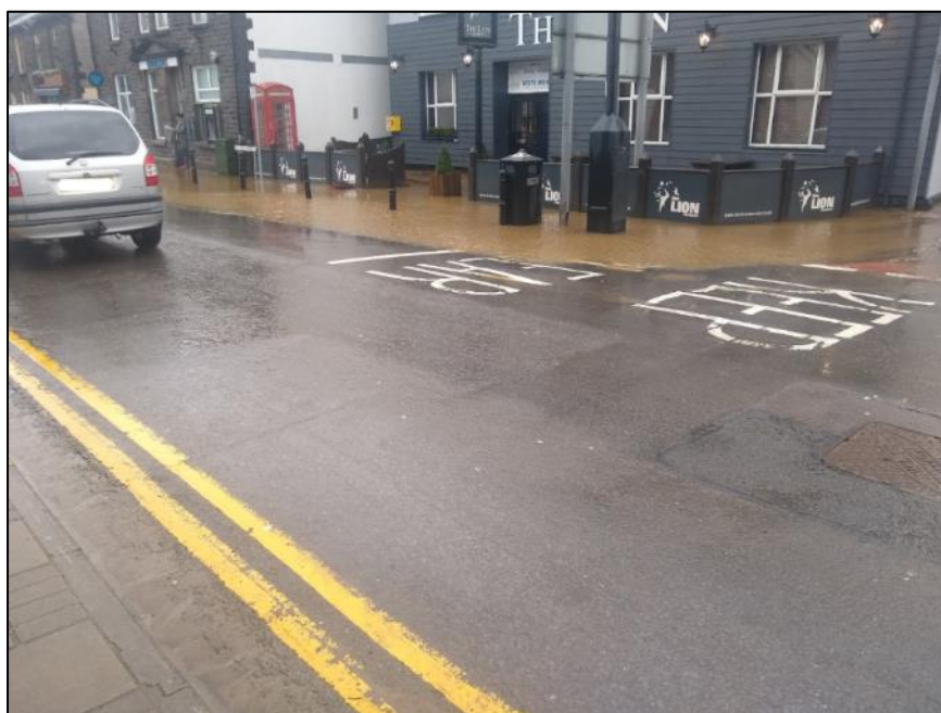
Figure 6: Surface water ponding along the A4061 High Street during Storm Dennis on 16 th February 2020 (image provided by resident)
