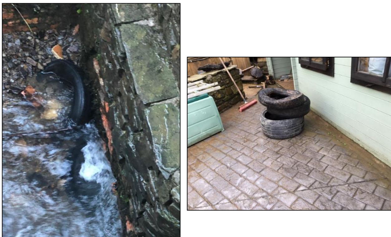
Figure 14: Evidence of debris, inclusive of tyres, causing a blockage to 'Culvert Inlet 2' during Storm Dennis (left) and evidence of the three tyres removed from the inlet by a resident (right) (images provided by resident)
