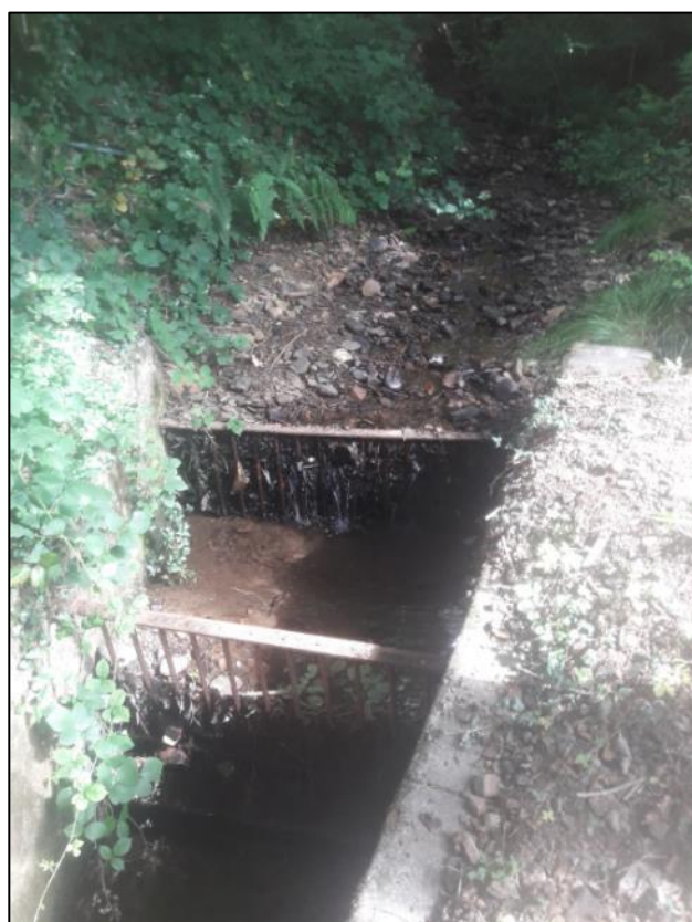
Figure 23: Photo of significant debris accumulation behind the upstream debris screens above 'Culvert Inlet 3' in the Nant Tyle-du watercourse (captured by a Council appointed contractor on 03/08/2020 during CCTV survey operations)
