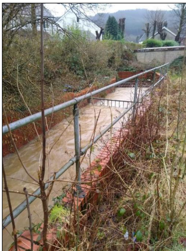
Figure 16: Column Street open channel and culvert inlet showing high flows (image provided by resident. Captured at 11am on 16th February 2020)
